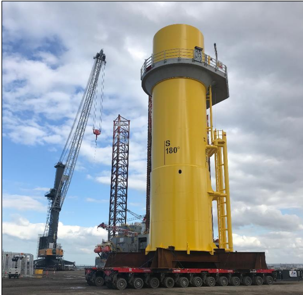
Figure 5: A Transition Piece being transported on a SPMT at Able Seaton Port
